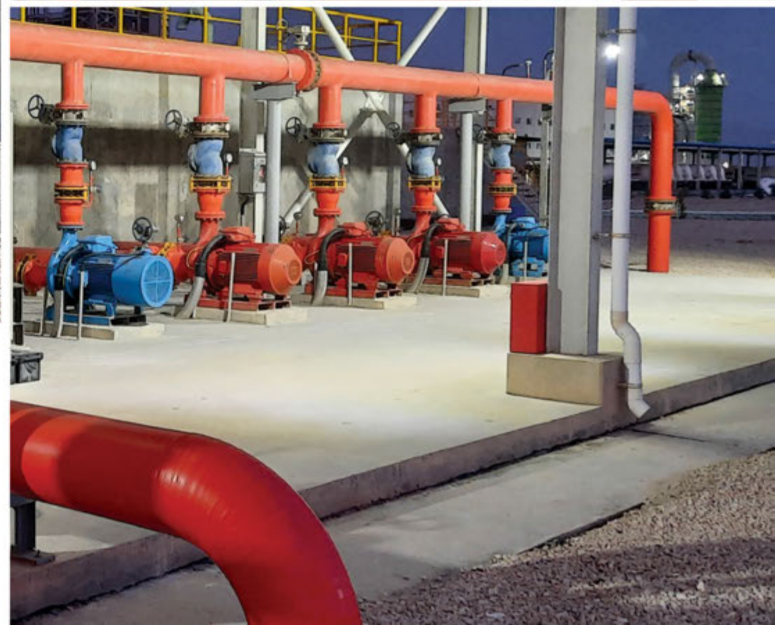
MOBARAKEH STEEL COMPLEX - COLOR WAREHOUSE Fire Alarm Systems (Simens & BW Technologies by Honeywell) Firefighting System (KCA Italy) ESFAHAN - IRAN, 2018 - 2020, PC
